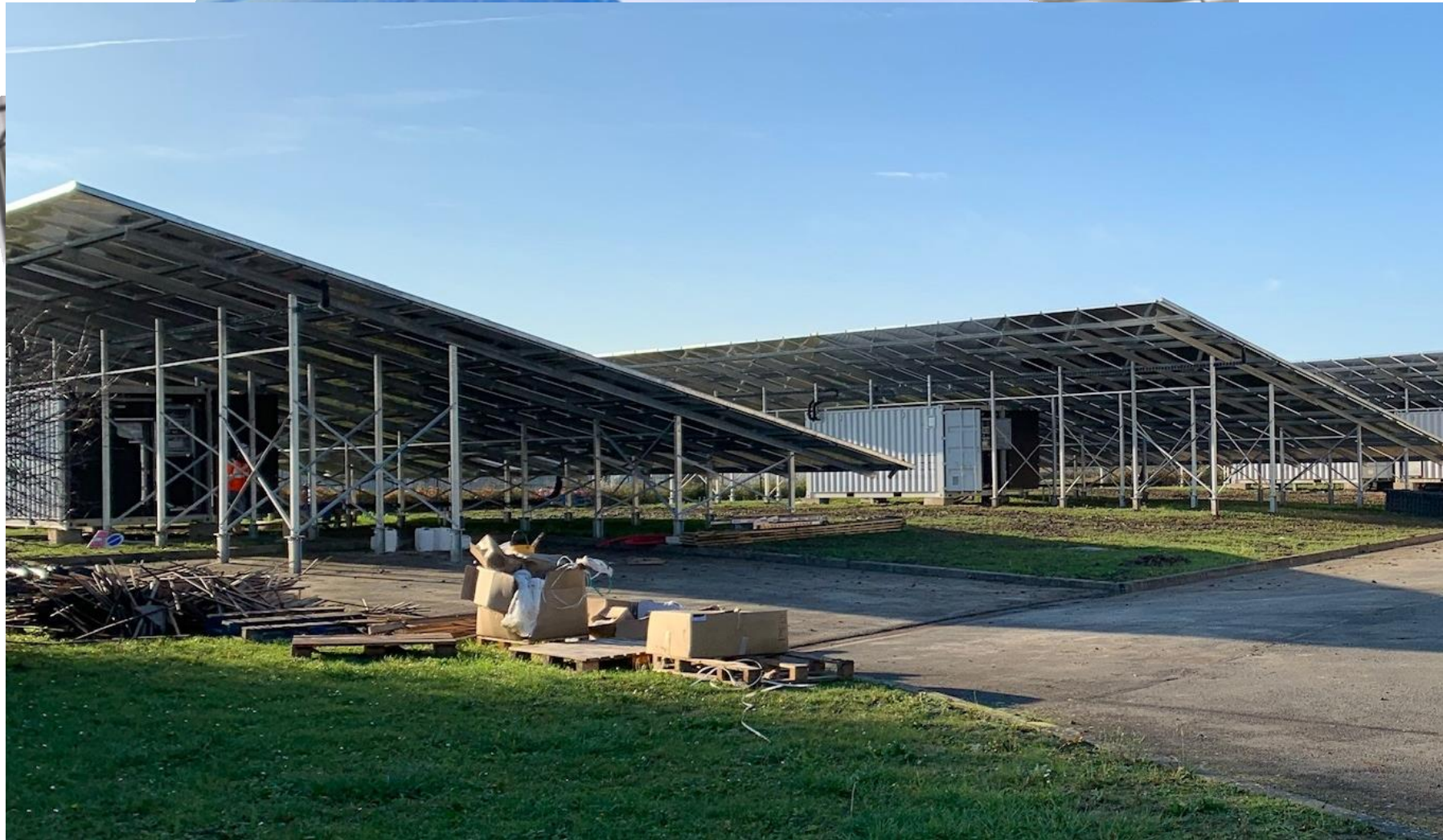
Drain-back solutions prefabricated in containers: Sunoptimo, Belgium
