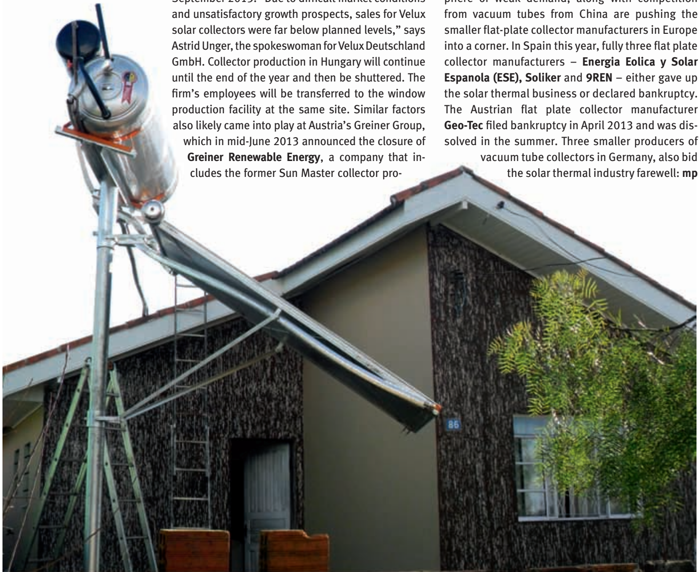
Surprising look: a 200 l solar water heater installed on a metal pole supplying the hot water of the family next door. The Brazilian company Soletrol won the tender of delivering 2,300 pole-mounted systems to COPEL, the local utility in the Brazilian state of Paraná.
