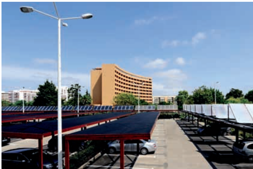
Space-saving installation of the collector field above the parking lot at the Crown Plaza Hotel at the Algarve in Portugal
